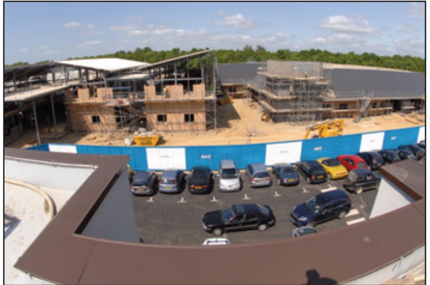
ABOVE: See how it grows...the new Mental Health Unit is taking shape fast.
